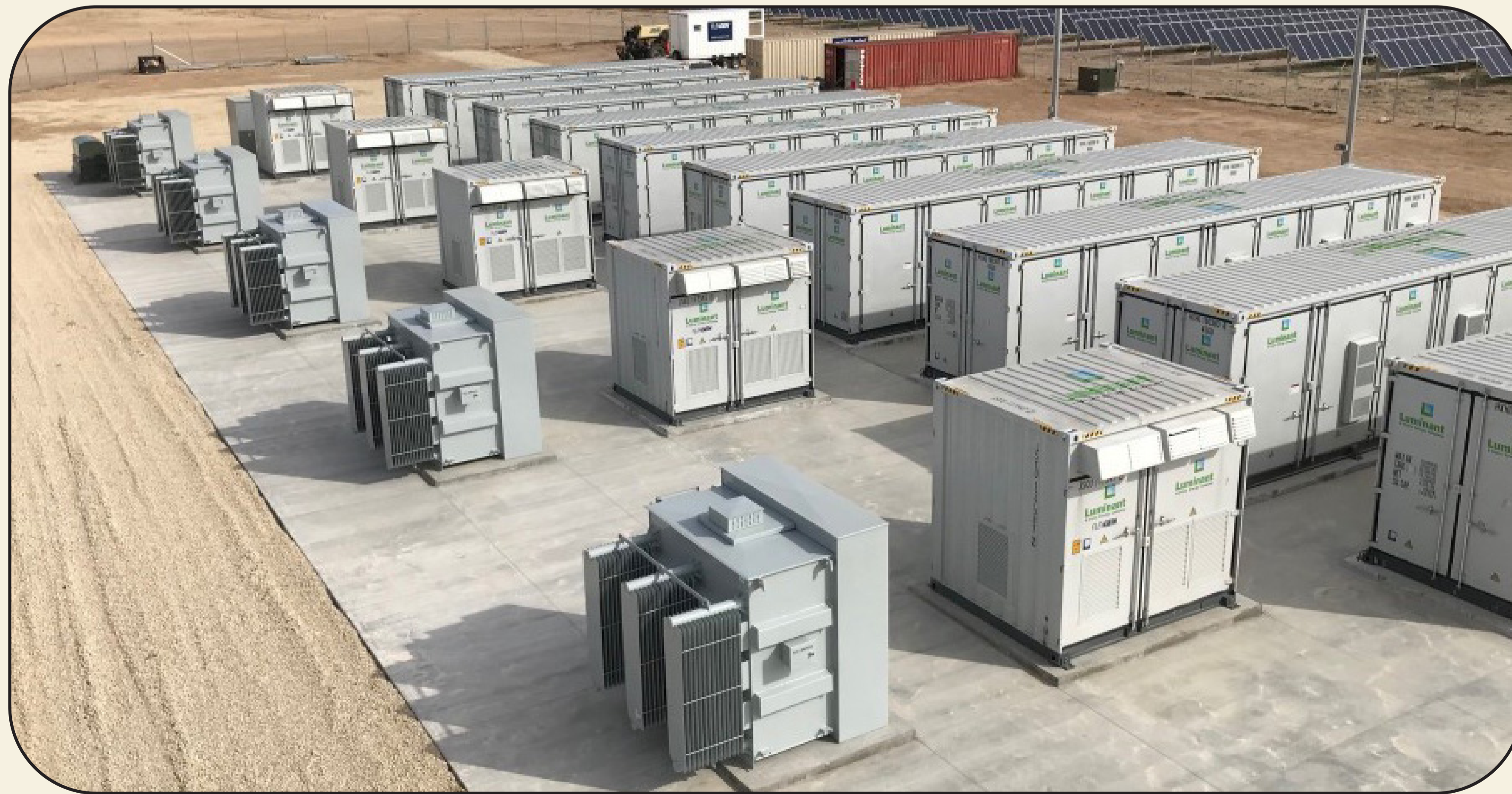
BATTERY ENERGY STORAGE PROJECT - EXAMPLE OF BATTERIES
